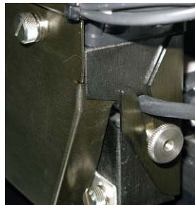
Figure 7-67: UV-lamp cable after replacing the assembly
